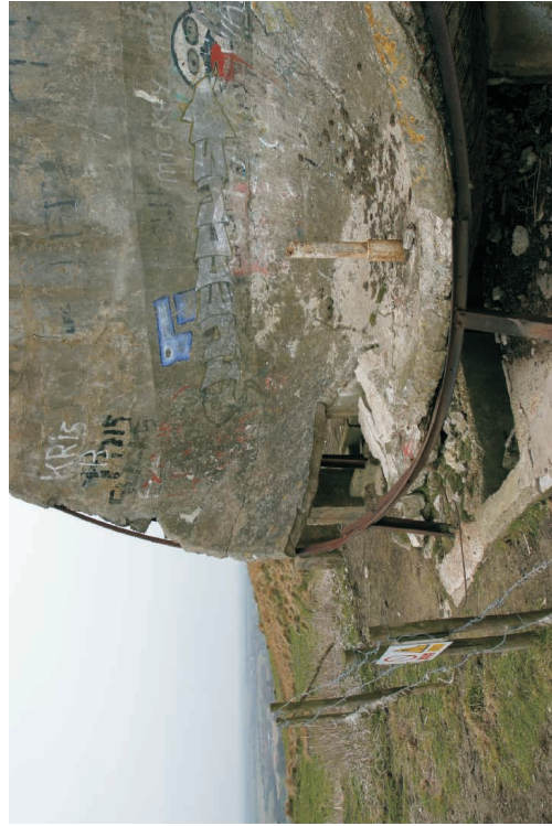
View of inside of Sound Mirror showing damage and decay
