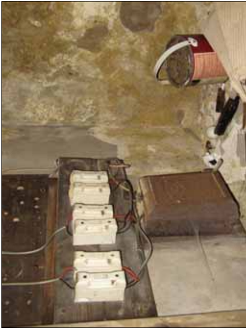
Plate 12: Possible circuit breakers in bunker
