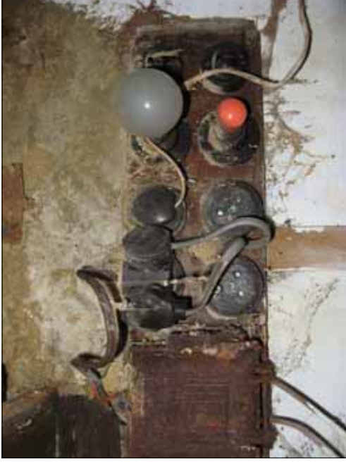
Plate 14: Bunker electrical fitting
