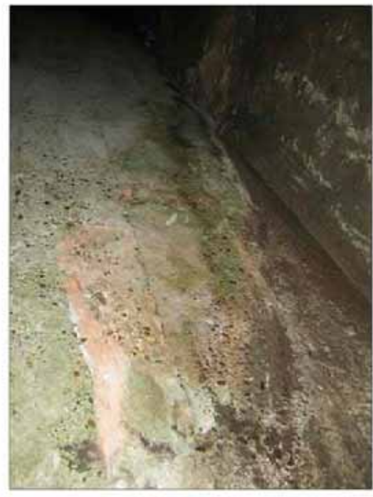
Plate 6: View of possible nail holes in wall inside shelter
