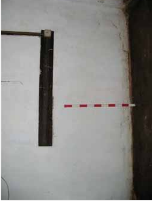
Plate 13: Bunker switch board
