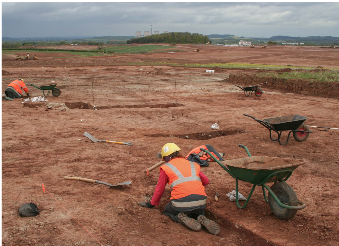
Plate 2.24 Looking north-east from Seven Geaves to King St Plantation (the site offices occupy the area where the King St Plantation excavations had taken place)
